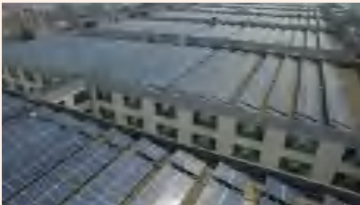
Factory roof solar photovoltaic panels
